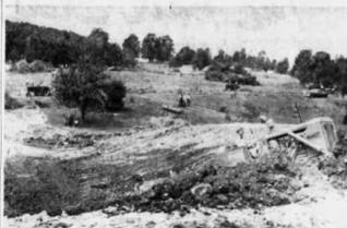
ONE-DAY POND—A bulldozer is used to construct a 300,000 gallon stock water pond, and other machinery clears and flows land of the conservation field day yesterday on the Mortimer Brooks farm in Great Brook.
