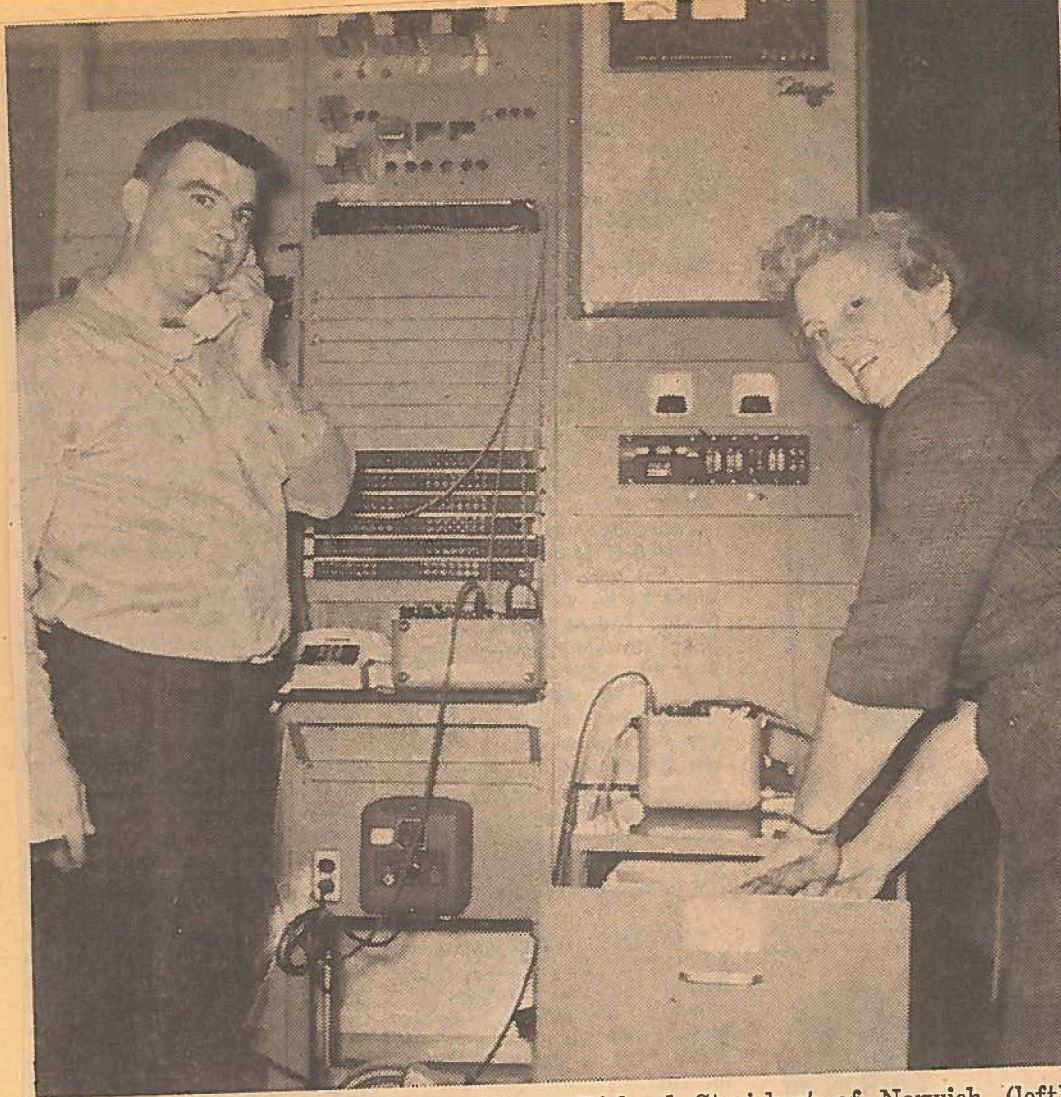
MORRIS GOES DIAL TOMORROW — Richard Streichert of Norwich (left) makes a final check of the new switchboard, and Mrs. Ceylon Decker checks the back room file of the new Chenango and Unadilla Telephone Co. facilities at Morris preparatory to the change-over at 12:01 a.m. Sunday to direct dialing.
