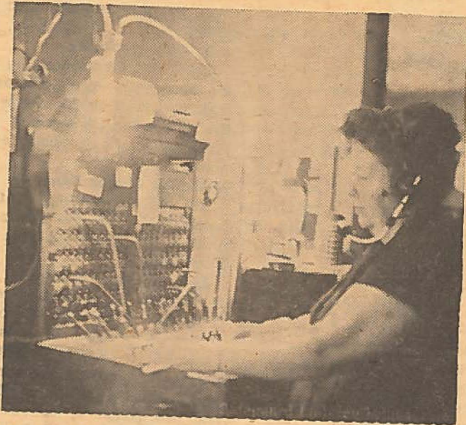
Mrs. Keith Stevens, substitute operator at the South New Berlin office is seen at the old switchboard shortly before it was replaced by a new board and new equipment.
